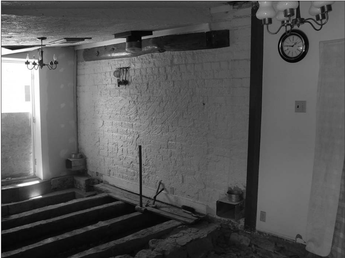
Figure 7. View of the central wall of the house in room block #3 from room block #4. Note the split log ceiling support bolted to the top of the wall, the walls bond pattern and adobe mud scratch coat can also be seen.
